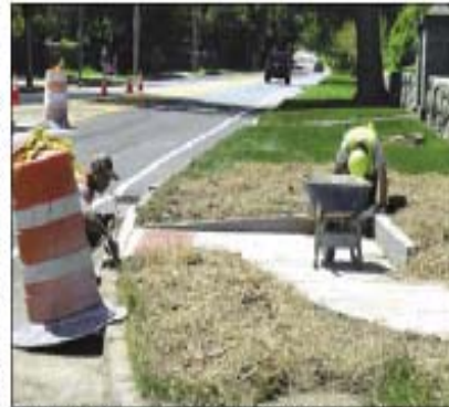
Workers are in the midst of completing a sidewalk access ramp to accompany a series of upgrades to the MS/HS portion of Boston Post Road. Photo: Christian Falcone
